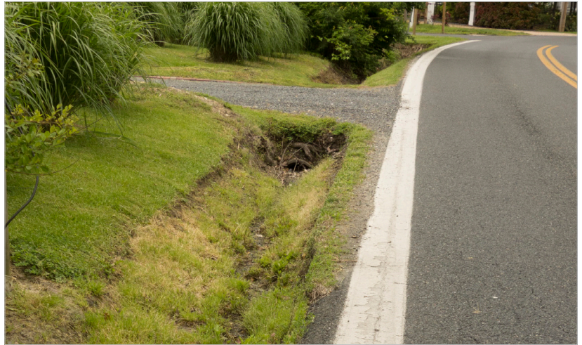
Figure 3.6 - Drainage ditch to convey stormwater runoff away from historic houses along the main road in the historic village of Royal Oak, Talbot County.
