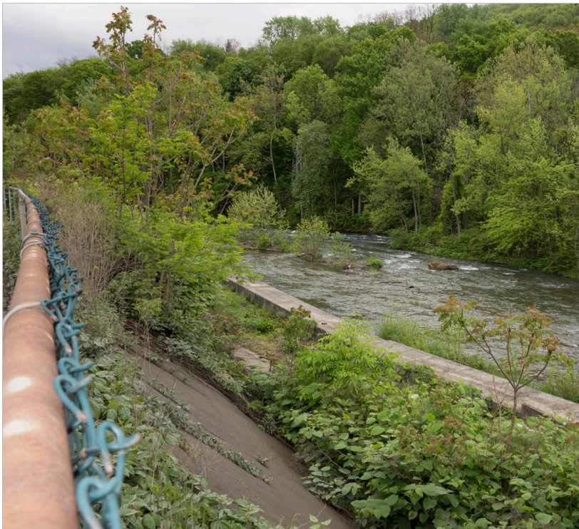
Figure 3.4 - Embankment with structural protections (concrete wall and embankment) to prevent erosion and stabilize the bank of the Potomac River. Westernport, Allegany County.
