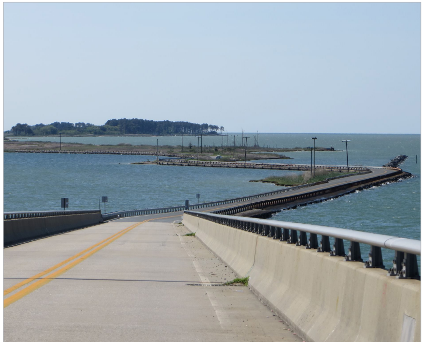
Figure 3.13 - Maintaining the main route to Taylors and Hoopers Islands could be challenging as the height of the Bay continues to increase and renders portions of the road impassable. Dorchester County.
