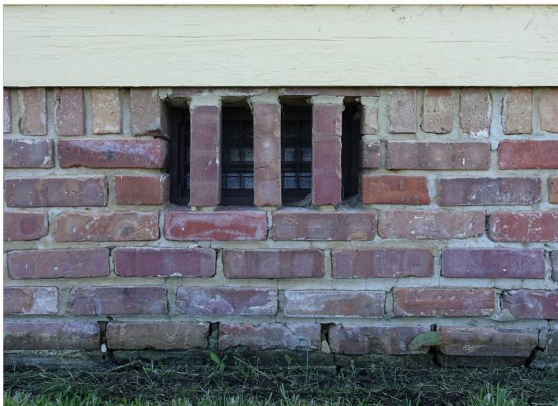
Figure 3.19 - The brick headers that conceal flood vents reduce the opening size of the vent, and may impede the flow of floodwaters out of the crawlspace. Whitehaven, Wicomico County.
