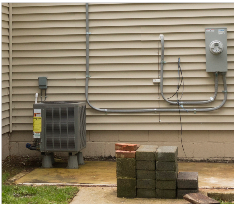
Figure 3.16 - Elevating mechanical and electrical equipment above the BFE is a basic improvement that may prevent the need for replacement in the event of a flood. Shady Side, Anne Arundel County.
