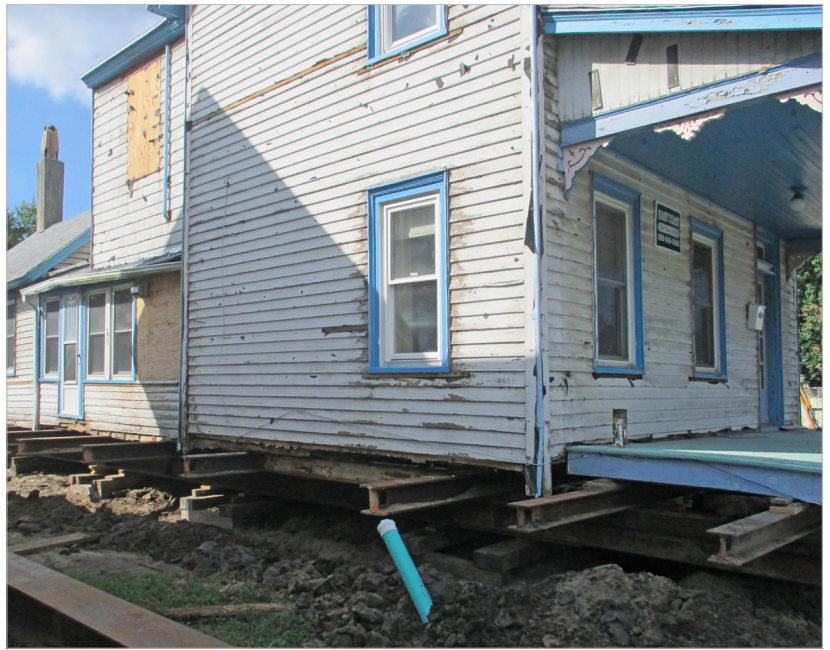
Figure 3.23 - Historic house on cribbing with a cradle of steel I-beams to stabilize the structure in preparation for relocation. Lewes, Delaware.
