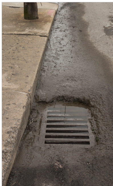
Figure 3.11 - Utility infrastructure improvements can be challenging to fund for small municipalities. Westernport, Allegany County.
