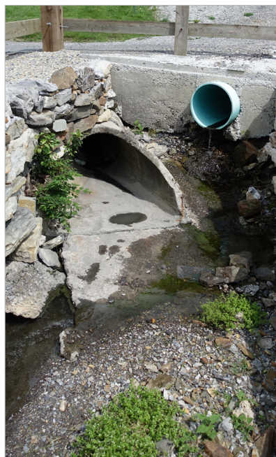
Figure 3.12 - An old outfall (left) and a potentially unpermitted discharge from a nearby property (center) that discharges into a ditch which could be retrofitted to allow for a stormwater filtration best management practice such as bioretention a swale, or a manufactured filtration device to improve water quality downstream. Williamsport, Washington County.
