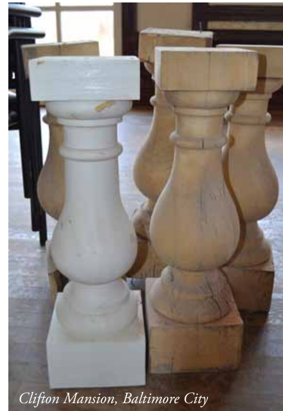
Easement program review of proposed work ensures that historic building elements are not lost and that missing or deteriorated elements are replaced to match, as shown above. Where railing components were missing, the new balusters (at left) were fabricated to exactly match the existing historic balusters (at right).
